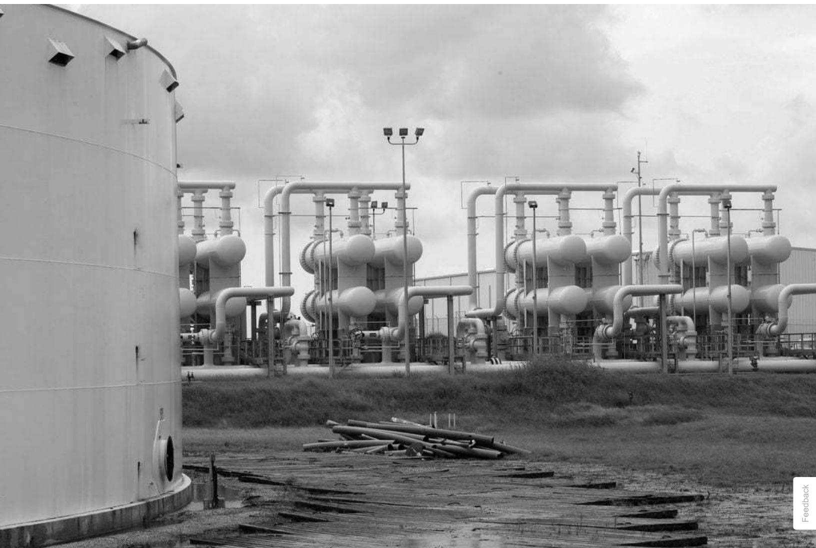
An oil storage tank and crude oil pipeline equipment is seen during a tour by the Department of Energy at the Strategic Petroleum Reserve in Freeport, Texas, U.S. June 9, 2016. REUTERS/Richard Carson Acquire Licensing Rights
